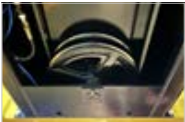
High end pulley and cable
